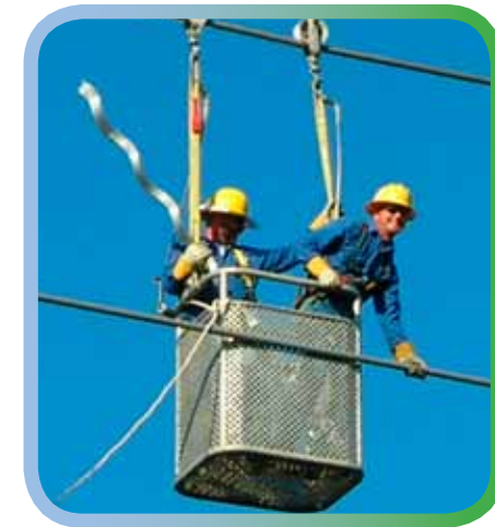
The transmission and distribution system carries electricity from LCEC power suppliers to customers.
