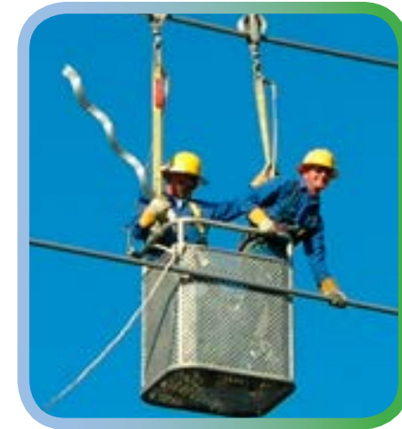
The transmission and distribution system carries electricity from LCEC power suppliers to customers.
